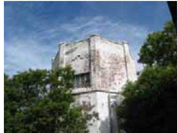
Figure 17: A. L. Cole Pump House at west side of Senator Buckwold Bridge.
