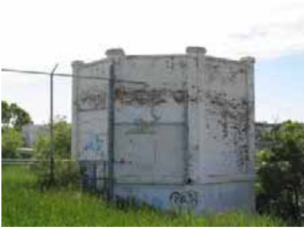
Figure 26: Existing A. L. Cole Pump House
