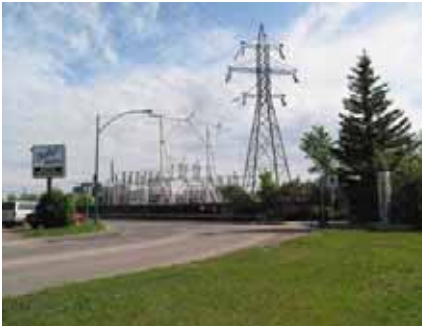
Figure 24: Existing electrical substation at south end of Avenue C looking east from Spadina Crescent West.
