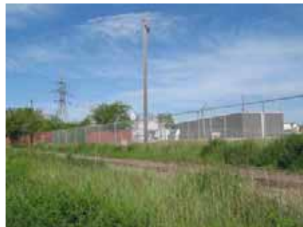
Figure 25: Existing electrical substation at south end of Avenue C looking north from future Spadina Crescent extension.
